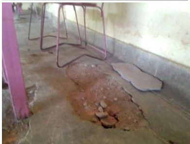
A school where the floor is planned to be repaired - Wayamba / Ibi / Manapaya Pri School.
